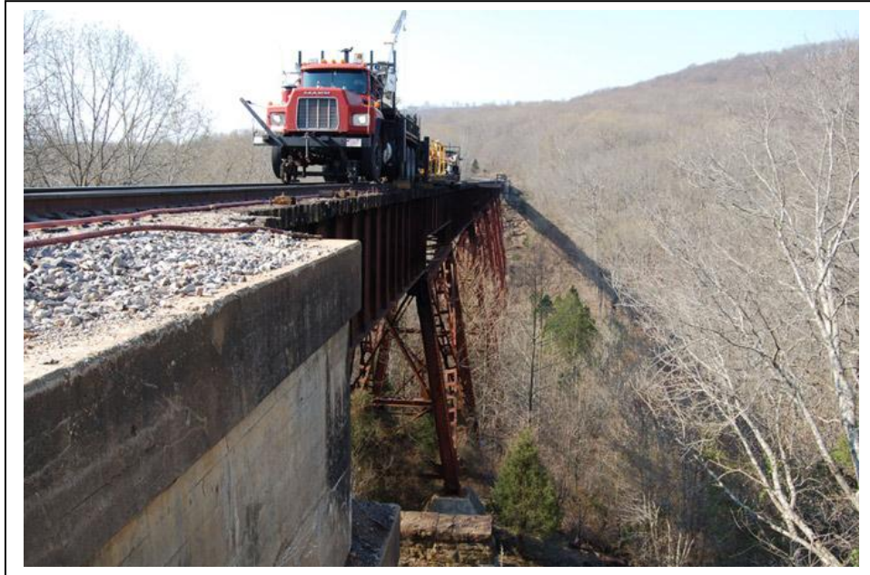
Workers use a rail-mounted truck with boom hoist to re-tie the 101 year-old Frisco Trestle.
